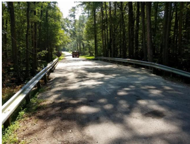
The Route 638/Mill Creek Road bridge over Burnt Mill Swamp in Isle of Wight County recently reopened to traffic after a full beam replacement. Photo: Virginia Department of Transportation
