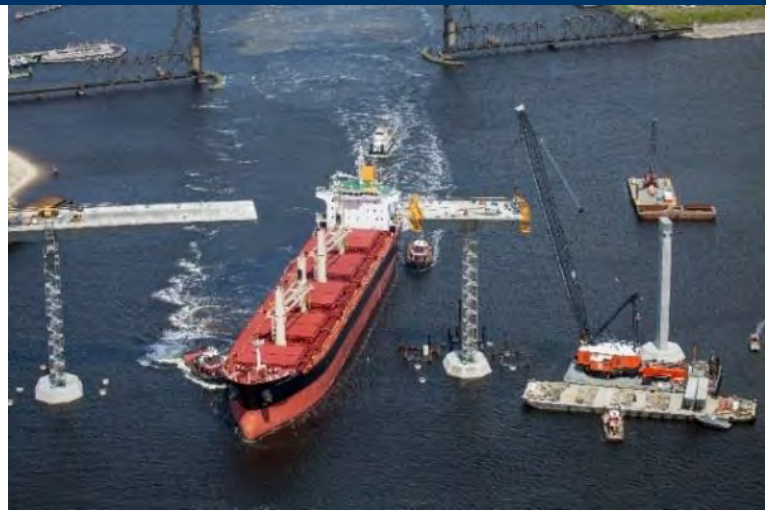
Figure 4.5.1.d. Construction operations over active navigable channel on Southern Branch of Elizabeth River by LMB team member.
