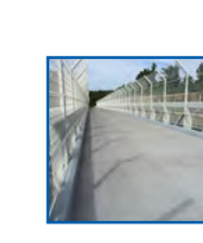
Bridge Roof No Roof
